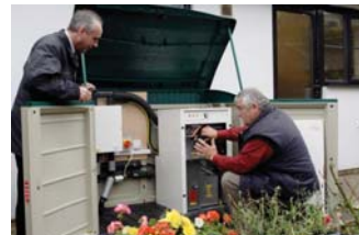
■ Simon Waters, left, and Tony Trolley, right, from Carrick Housing pictured with a Calorex ground-source heat pump unit.
