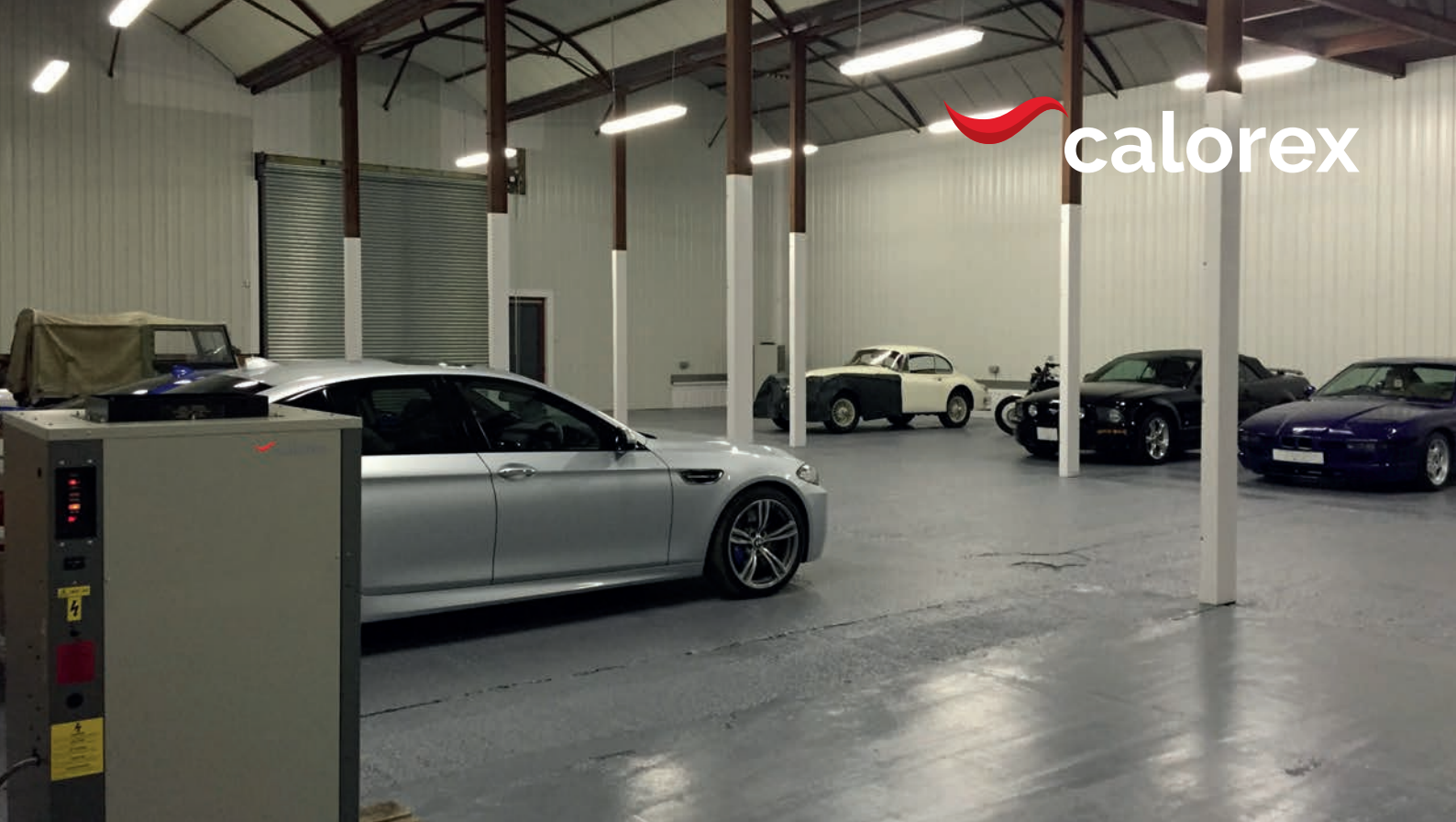
Calorex DH 150 in situ at TMS Car Storage
